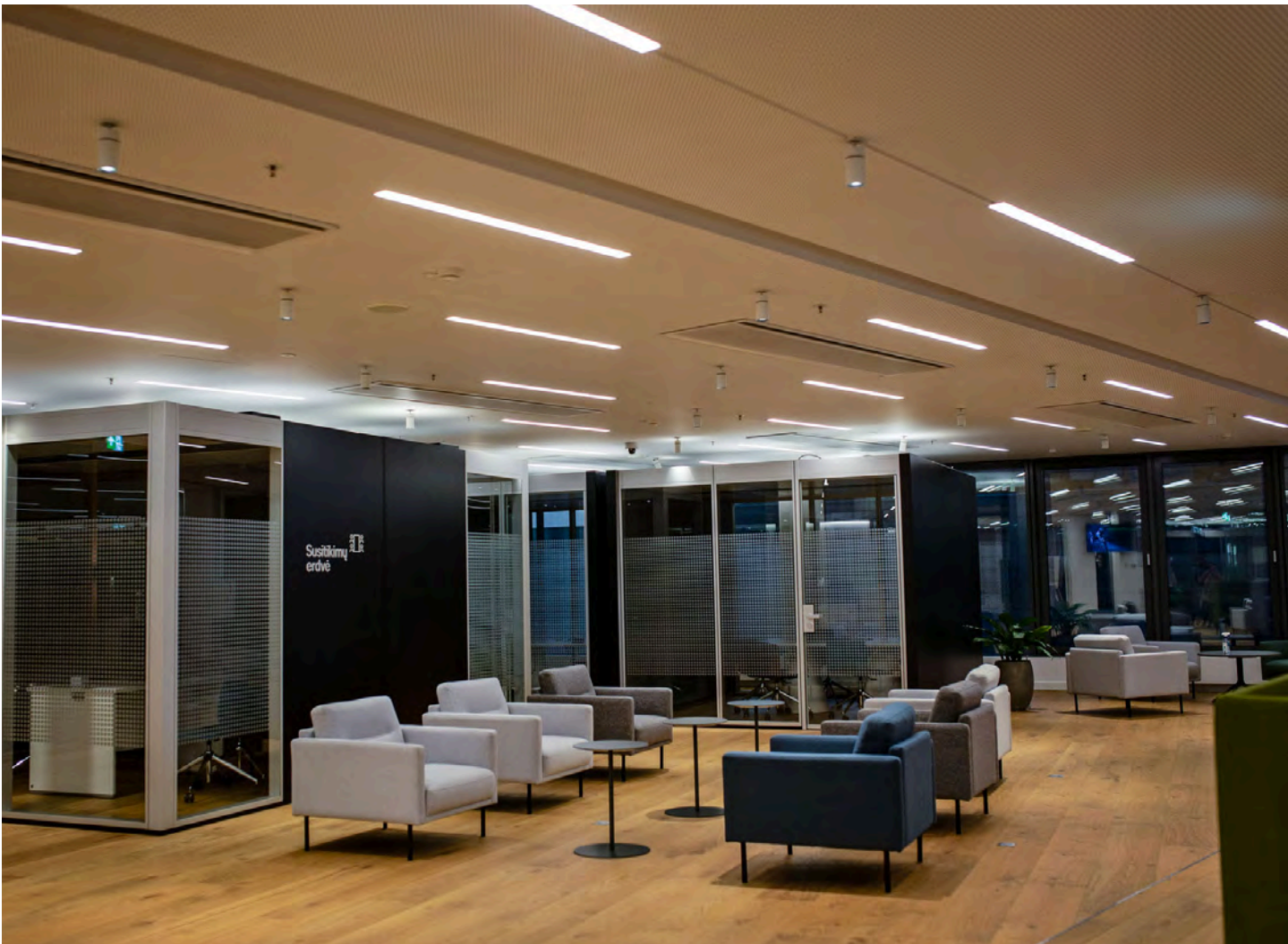
The modern lighting fixtures for the SEB Bank premises were manufactured according to a unique design with specific technical parameters and dimensions for maximum visual comfort.
